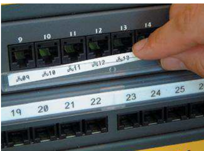
Punch Block & Patch Panel Labels
